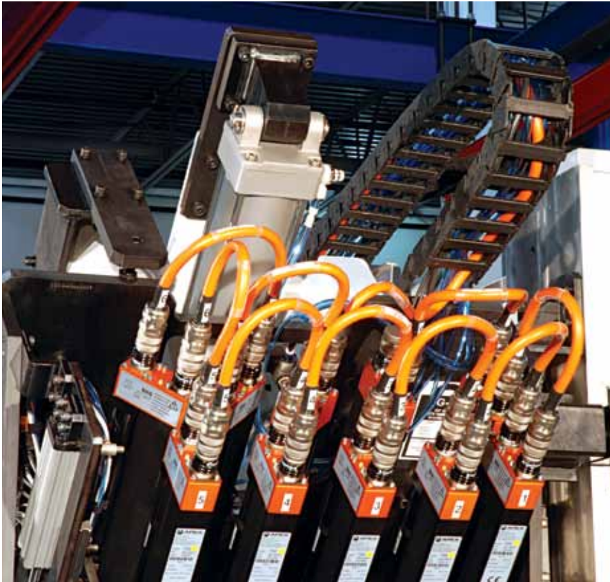
Shown above is a ten Intelligent spindle application with nine jumper cables and a single field cable that terminates at the power distribution box.
